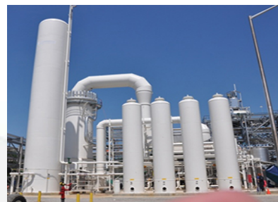
8,500 Kg/day (4,000 Nm 3 /h plant Location: USA
